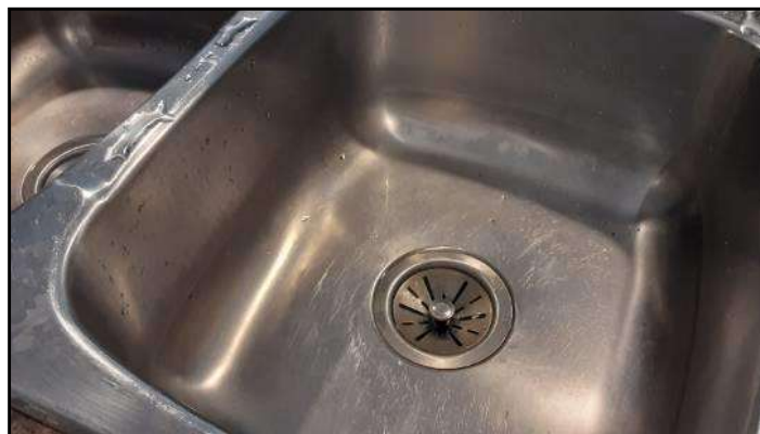
61. Drain stop ineffective
