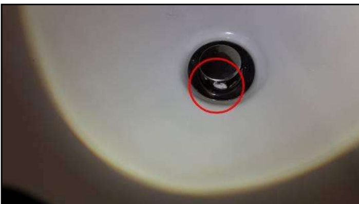
62. Drain stop ineffective
