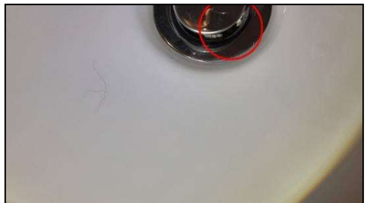
63. Drain stop ineffective
