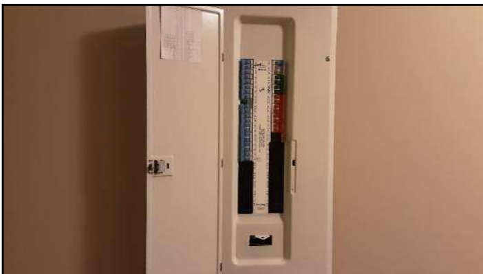
16. General view of the Electrical panel
