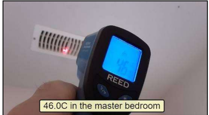
13. Furnace air flow and temperature taken at the
