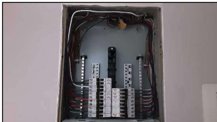
9. General view of the Electrical panel
