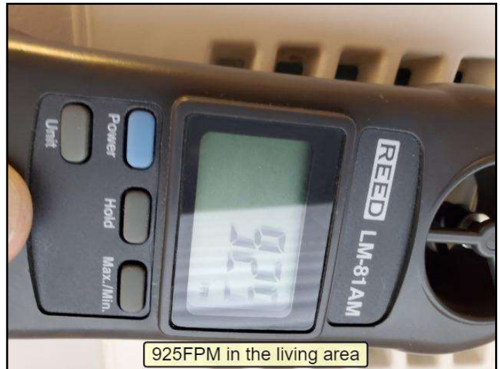
15. Furnace air flow and temperature taken at the
