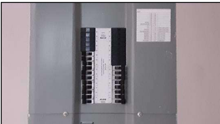
8. General view of the Electrical panel
